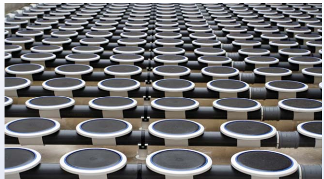
A grid of ABS Nopon aeration diffusers
